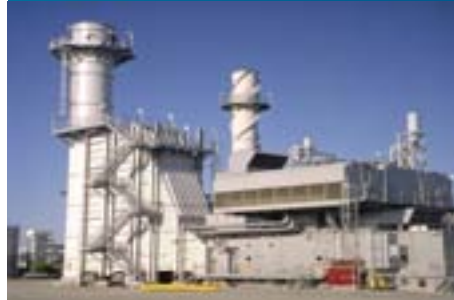
Simple cycle SCR and CO system on LM 6000 gas turbine
