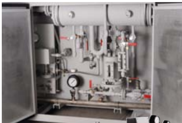
Fluid system sub-assemblies with piping, vessels and instruments.
