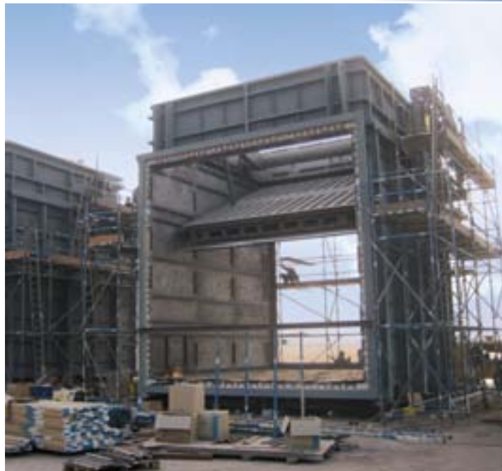
Qatar – 9F toggle linkage mechanism installed on a diverter damper.
