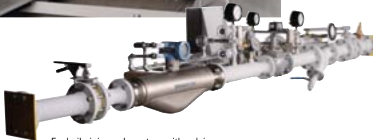
Fuel oil piping sub-system with valving and instrumentation for measuring flow, temperature and pressure
