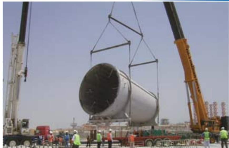
Qatar – SGT5-4000F exhaust diffuser
