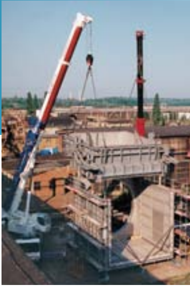
Argentina – pre-assembly of SGT5-4000F diverter for functional testing
