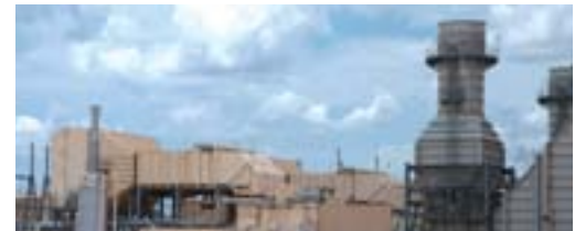
USA – 7FA exhaust system
